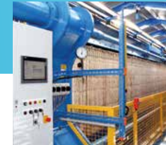
Filter press & Decanter centrifuge (SLUDGE MANAGEMENT)
