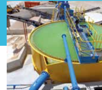
AquaCycle (PRIMARY STAGE WATER TREATMENT & RECYCLING)
